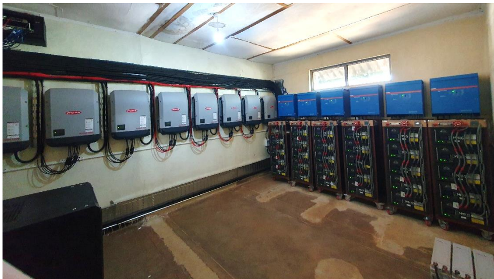
Solar room with inverters and batteries
