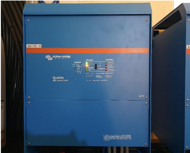
Victron Quattro battery inverter/charger
