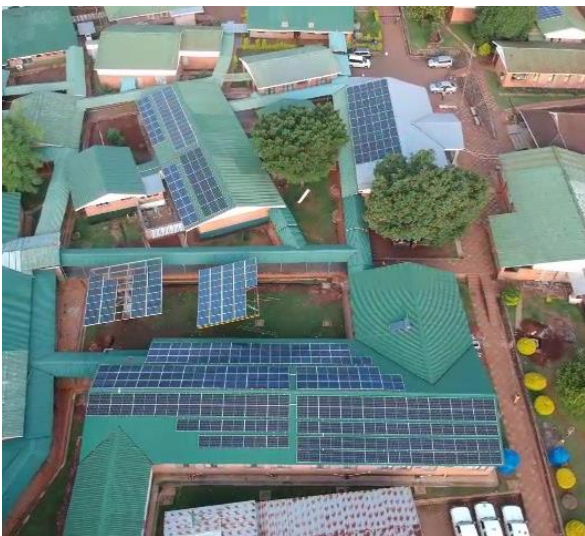
Solar panel arrays in North and East/West direction for energy during all day hours
