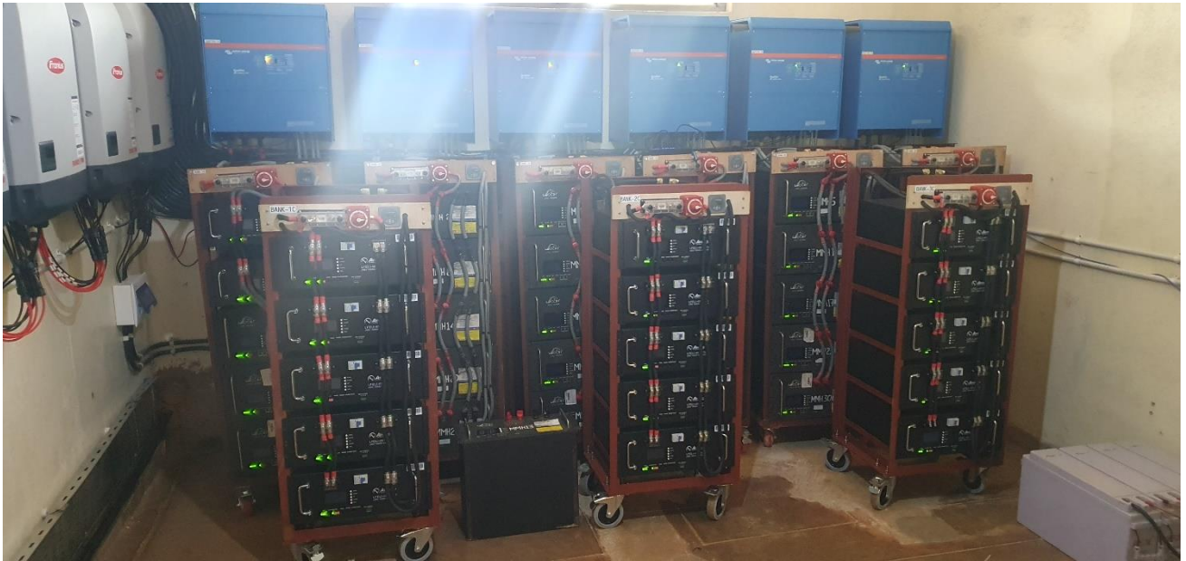
45 Lithium-ion batteries, across 9 banks in the power house at MMH
