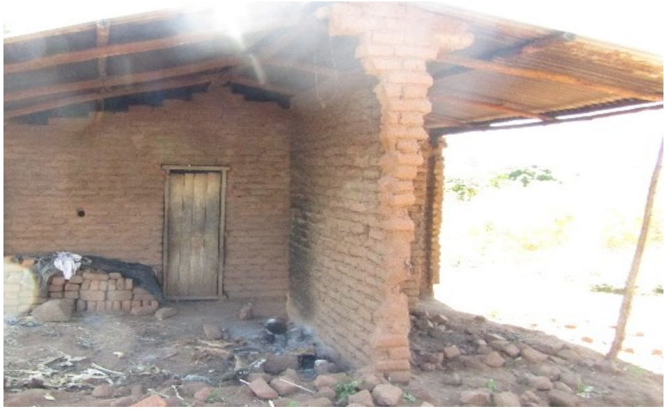
House at Khoviwa after floods
